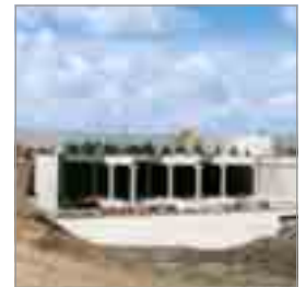
North Meadowvale Reservoir and Pump Station, Ontario (CA), 2006
